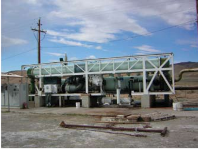
Figure 1. 2MW geothermal power plant that provides electricity for the biodiesel plant.
